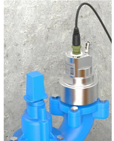
Figure 28. Example of a Hydrophone-2 installation
